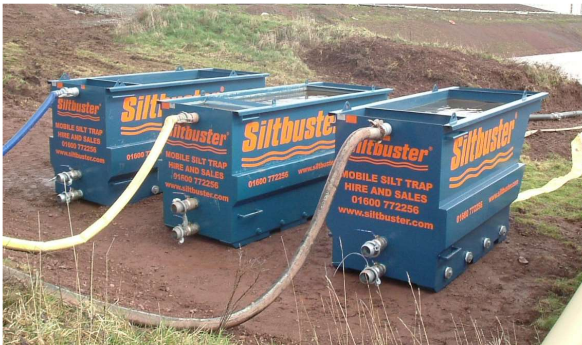
Figure 5.3 Temporary site settlement tanks (Source: Siltbuster)
